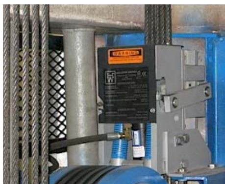
Fig. 2 Second Braking Mechanism on an Elevator in the City of Houston Code Enforcement Building
